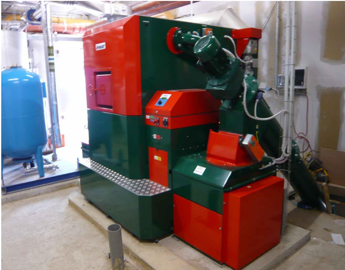
Obr. 3 Kotel Hamont catfire
